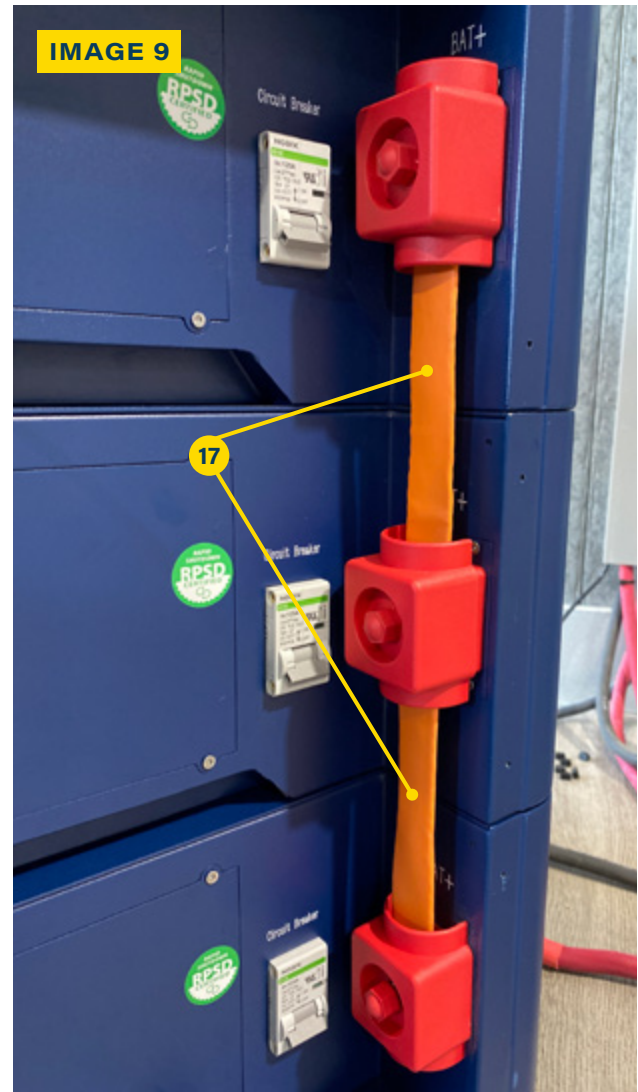
17 PARALLEL BATTERY CABLE
