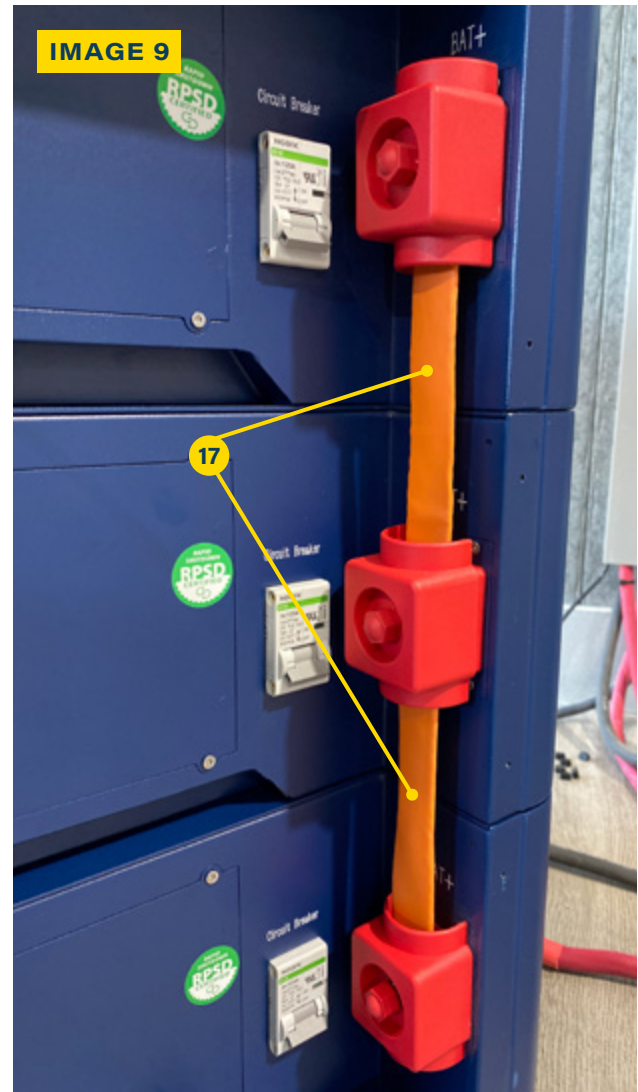
17 PARALLEL BATTERY CABLE
