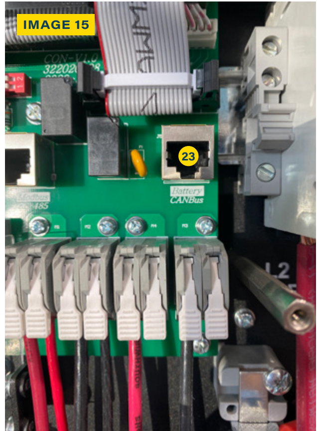
23 CANBUS PORT ON SOL-ARK INVERTER
