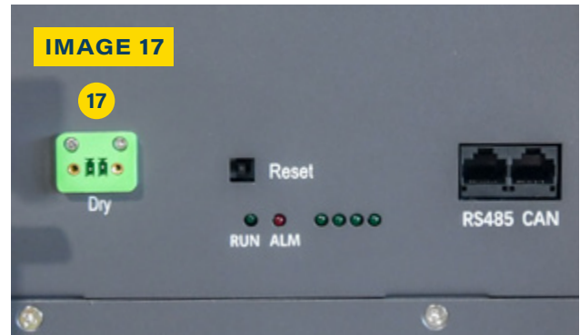
17 RAPID SHUTDOWN TERMINALS.
