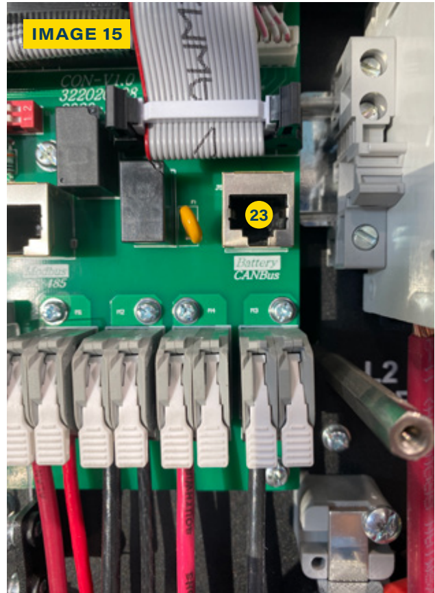
23 CANBUS PORT ON SOL-ARK INVERTER.
