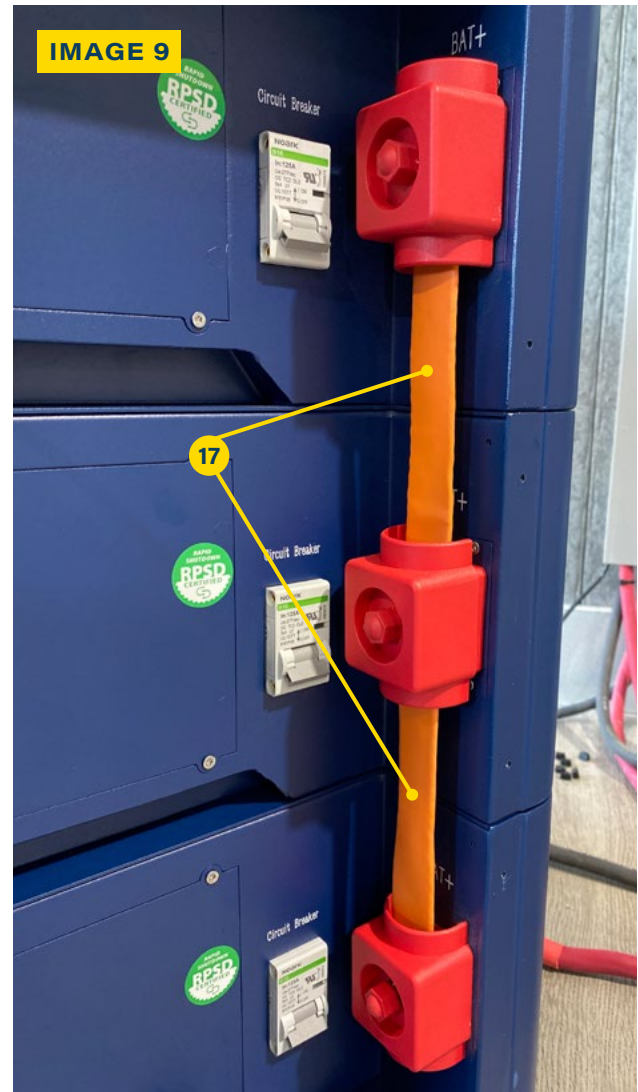
17 PARALLEL BATTERY CABLE
