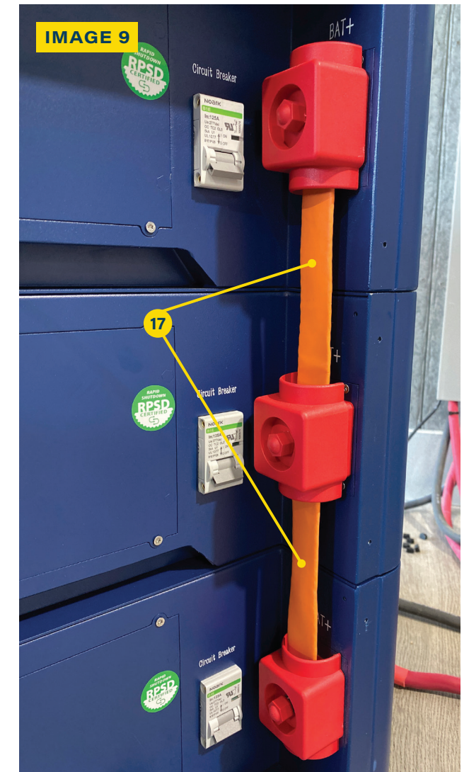
17 PARALLEL BATTERY CABLE
