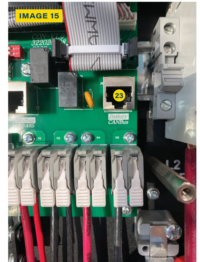
23 CANBUS PORT ON SOL-ARK INVERTER
