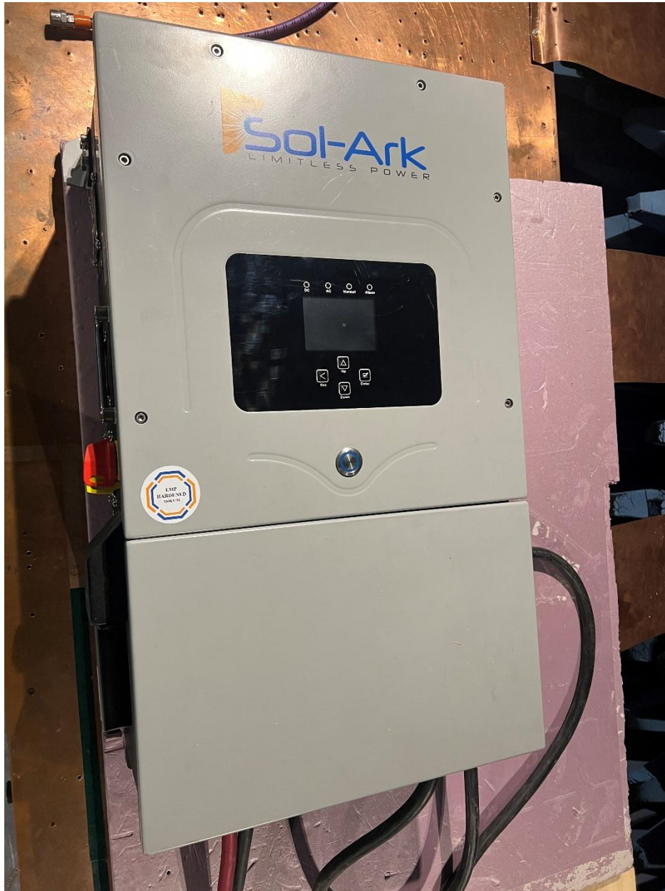
10 Support Equipment - Sol-Ark 12k-P
