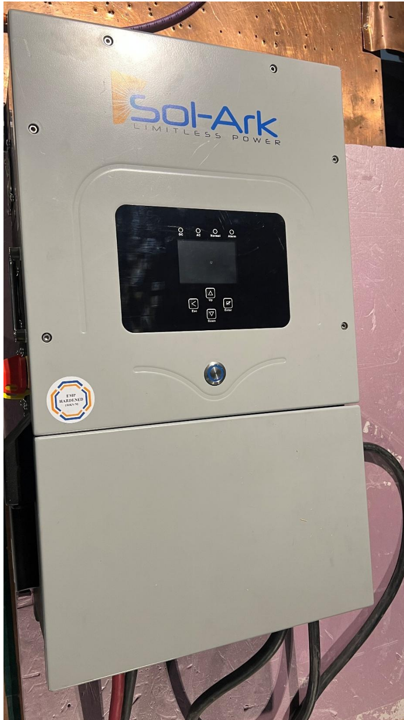
07 Support Equipment - Sol-Ark 12k-P
